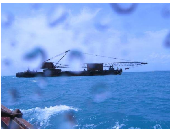
Figure 1: Photo showing large barge with crane observed at C1. (Photo taken -15 August 2014)
